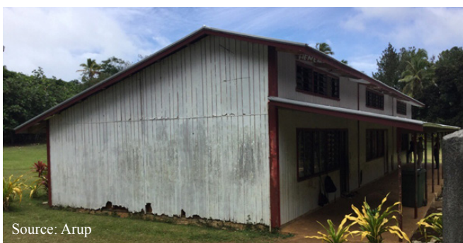
Source: Arup Standard engineered school designs developed in 1982 following Cyclone Isaac have been shown to withstand multiple intense storms, but require urgent maintenance to ensure their long term viability.
