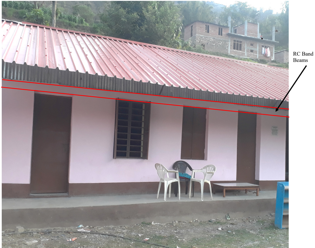
Horizontal ring beam installed in an LBM type school building in Nepal that was damaged (minor) after the 2015 Nepal earthquake (Photo from Nepal, Copyright: The World Bank)
