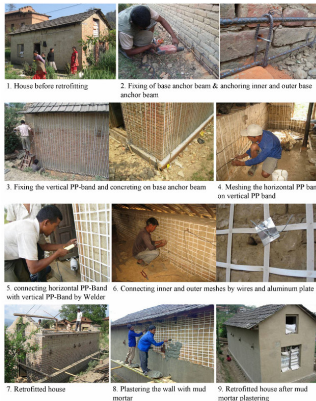
Example application procedure of PP band mesh in an adobe building (Reproduced from Sathiparan, 2015)
