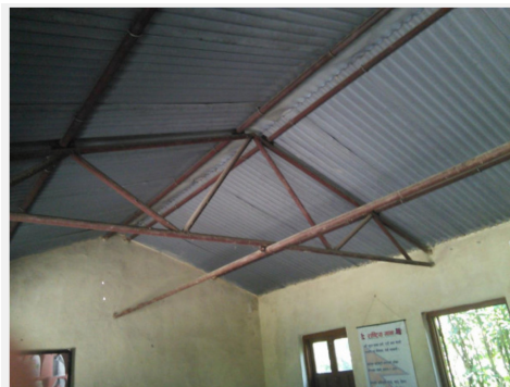
Light steel roof structure in an LBM school building in Nepal (Copyright: The World Bank).
