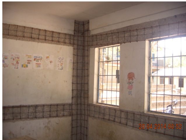
An UCM-URM4 type of LBM school building being strengthened using RC Splint and Bandage technique (Photo from Nepal, Credit: Sunil Kumar Yadav, MoE, Nepal).
